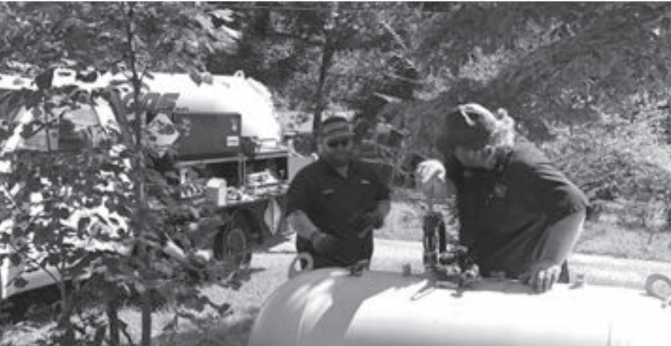
A new propane tank is installed at the Mentone American Legion.
